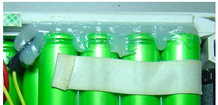
Excess silicone insulation can block safety vents
